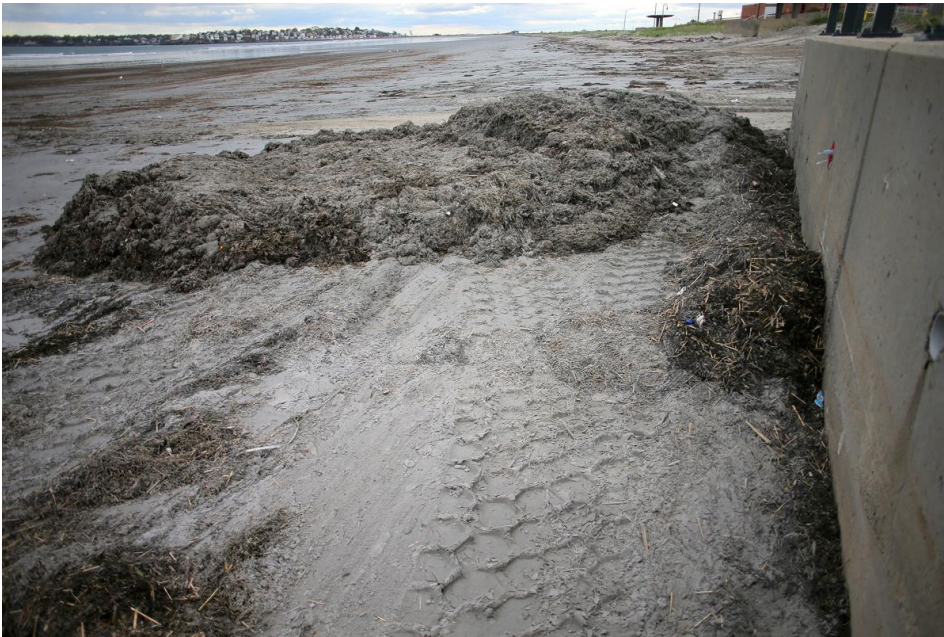
A pile of tidal debris has been pushed up against the seawall by heavy machinery. The debris is then trucked to a landfill.
